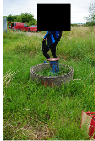
CMS monitoring well at leachate pumping station
